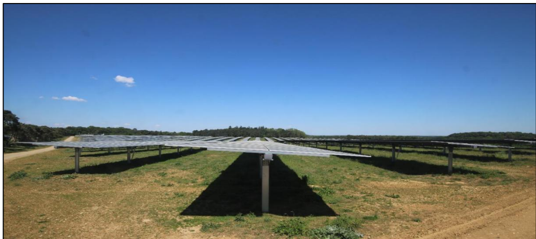
Plate 2 Typical Tracker Solar PV Panels in a Near Flat Orientation
