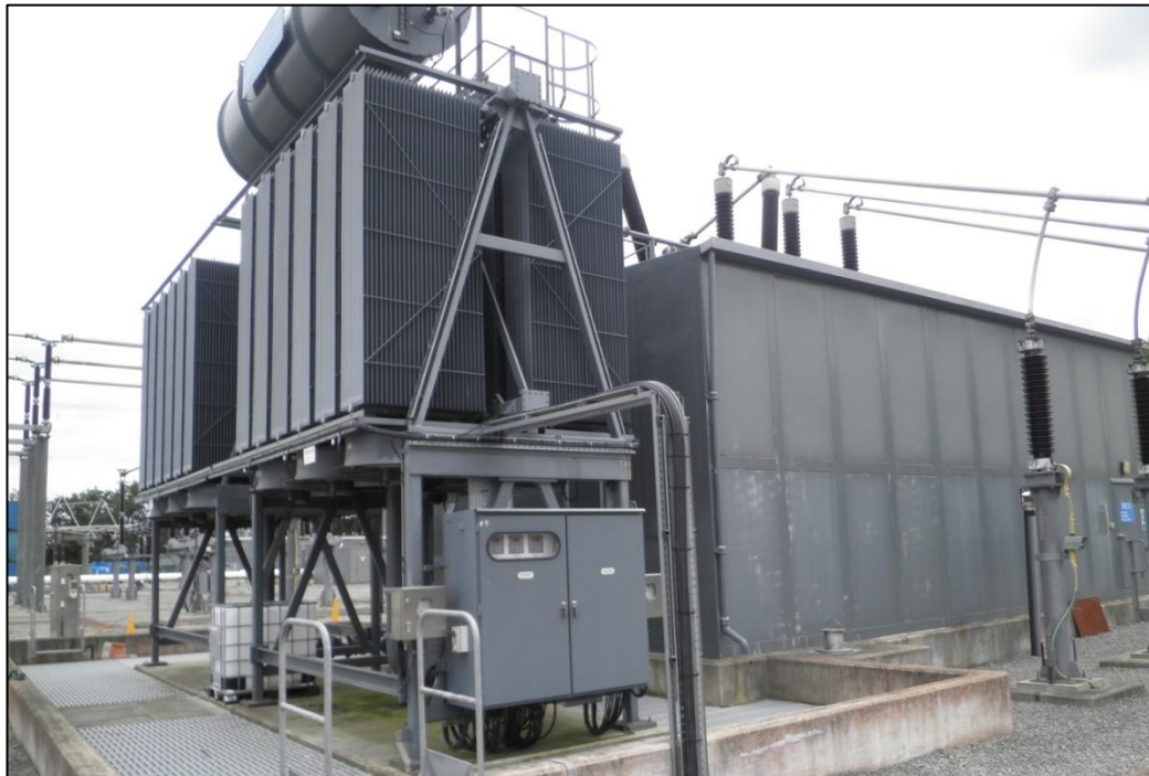
Plate 10 Air Insulated Substation
