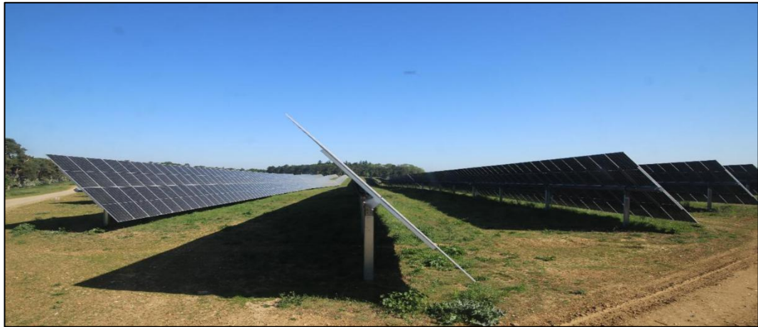
Plate 1 Typical Tracker Solar PV Panels in an Angled Orientation
