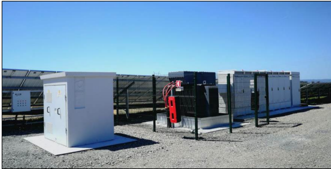
Plate 8 Typical Standalone Equipment Making Up a Conversion Unit
