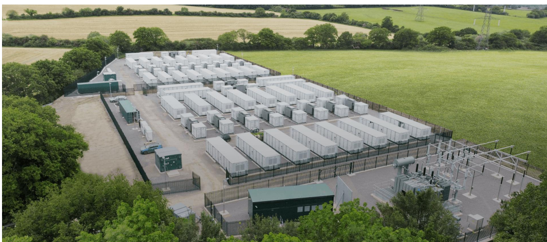
Plate 9 Typical Battery Energy Storage System
