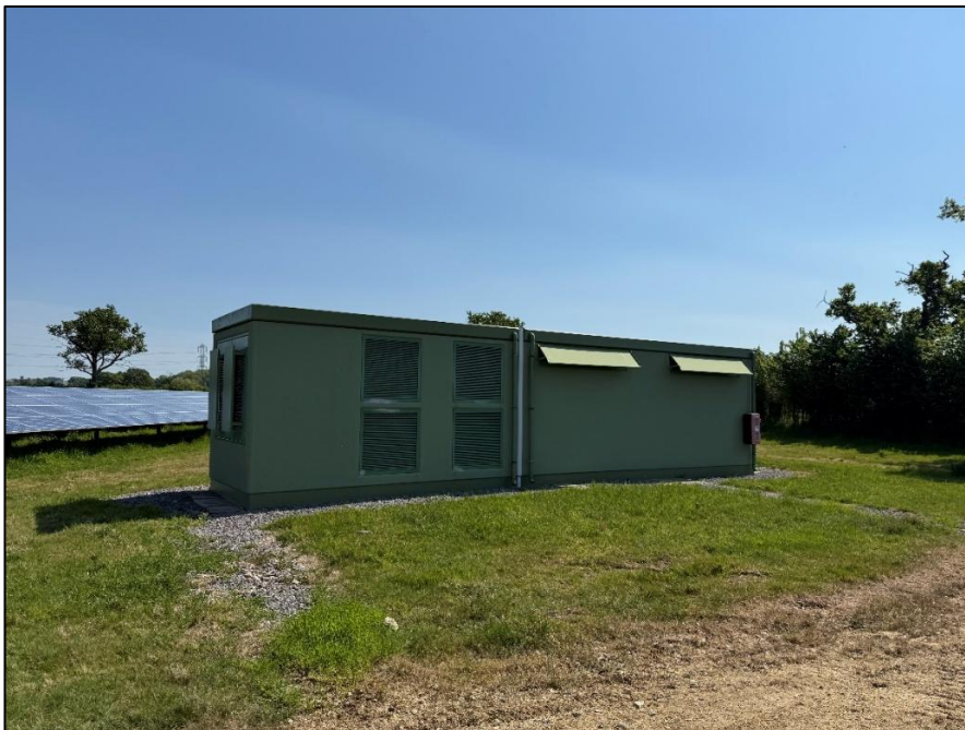
Plate 6 Typical Conversion Unit / 33kV Sub-distribution Switch Room
